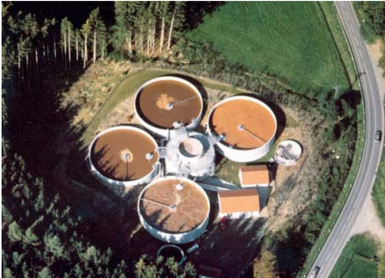
Four-basin AquaSBR system
