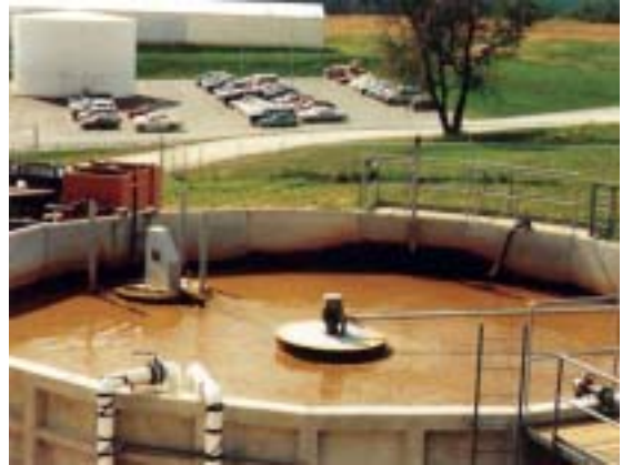
Dairy plant in Pennsylvania effectively treats waste with an AquaSBR system.
