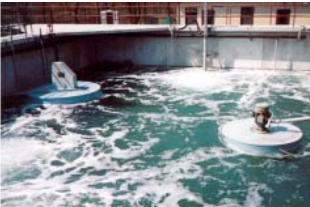
Domestic waste treatment with the AquaSBR system.
