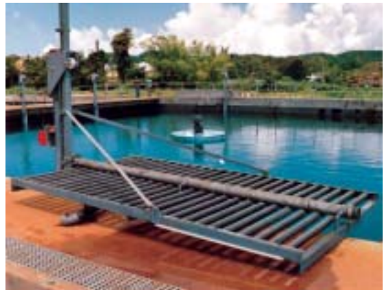
Diffusers easily retrieved at this pharmaceutical company in Puerto Rico.
