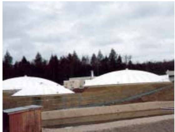
Covered tank AquaSBR system.
