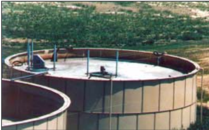
Single basin AquaSBR system measures 47" in diameter x 16' SWD
