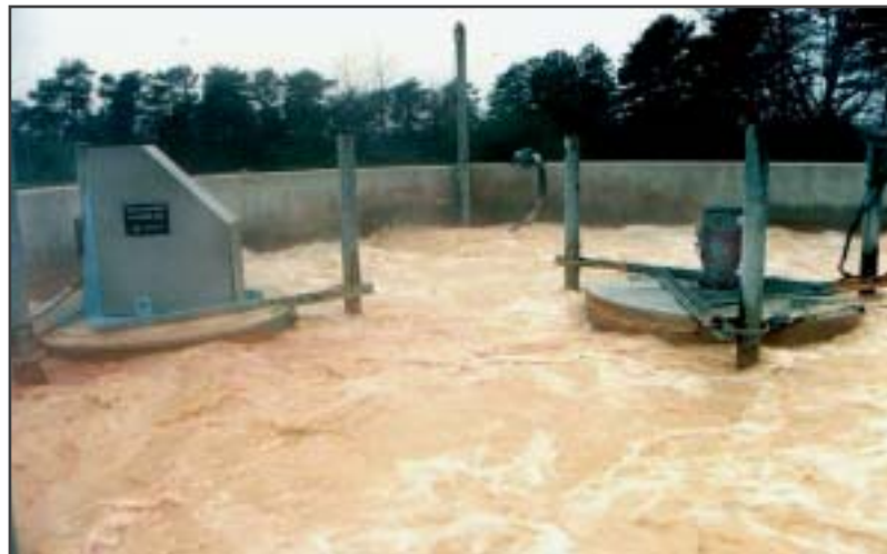
One of the AquaSBR basins in operation.
