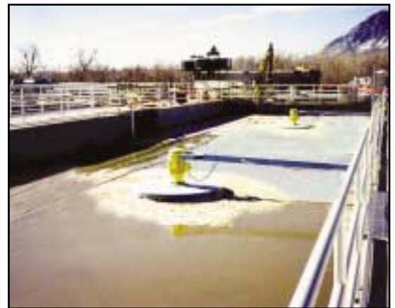
One of five anoxic basins utilizing AquaDDM mixers with a pivotal mooring arm.
