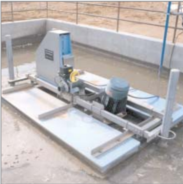
This AquaCAM-D ® unit treats domestic wastewater from an outlet mall in New Mexico.
